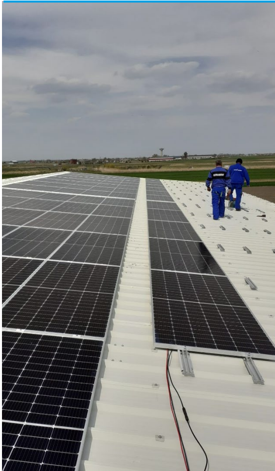
Photovoltaic plant in Romania.
